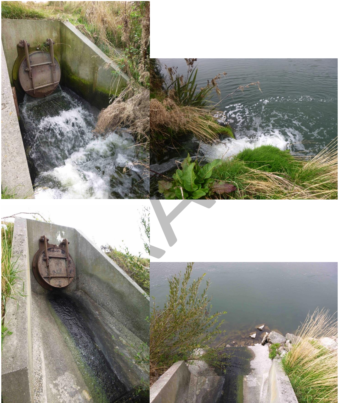
Figure 3. Gore Actiflo® plant outfall (top) and oxidation pond outfall (bottom), 6 March 2020.
