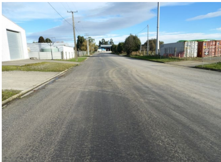
Photo 3 – Sediment build up along Aparima Street
