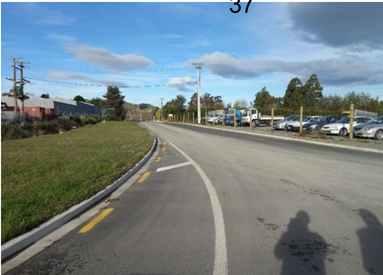
Photo 4 – Sediment build up along Falconer Road
