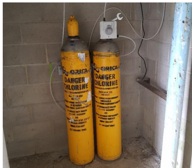
Figure 7: Chlorine Gas Storage
