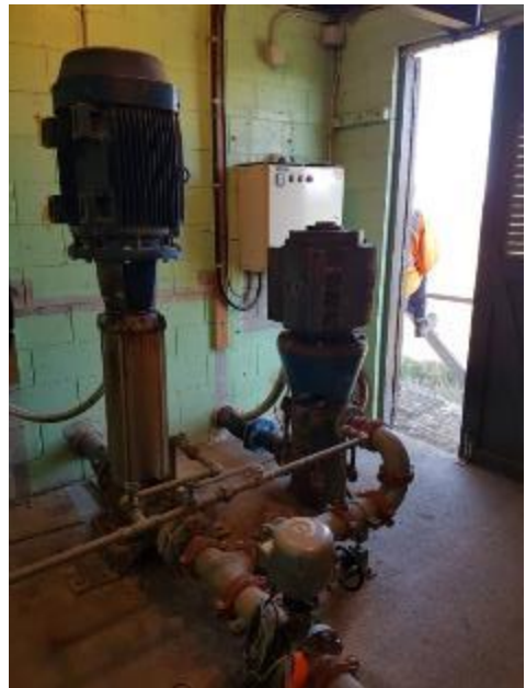
Figure 5. Pyramid Road Service (left) and backup pumps
