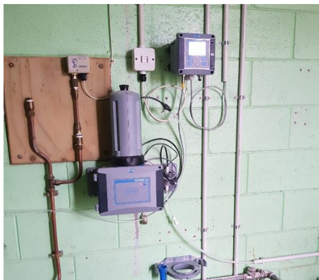
Figure 6: Chlorine Dosing and Online Turbidity Meter
