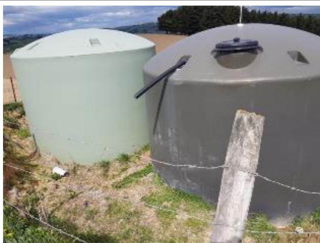
Figure 142: Pinnacle Rd Break tank
